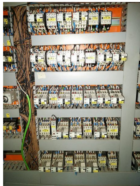
Typical "Relay Control" automation panel
